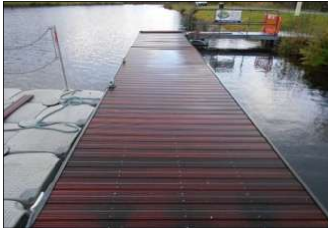
Before & after photos of pontoons: bearers had completely rotted.
