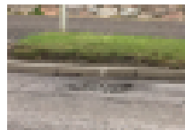
sunken drain cover at bus stop at Kilmallie Gardens
