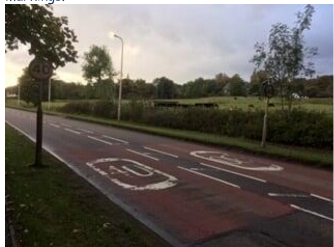
Poor road markings just past Ravenswood.
