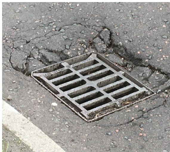
Sunken drain cover close to Kilmallie Gardens.
