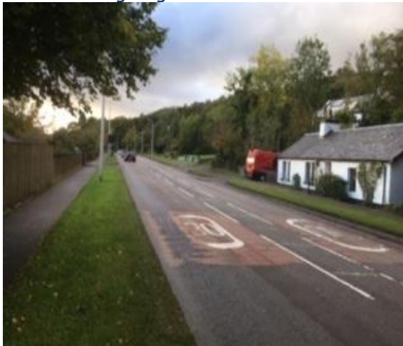
Corpach travelling West. Poor road markings.
