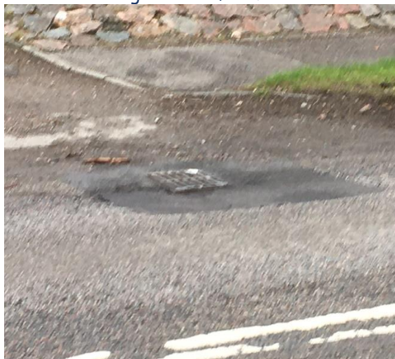
Sunken drain cover close to Kilmallie Gardens.
