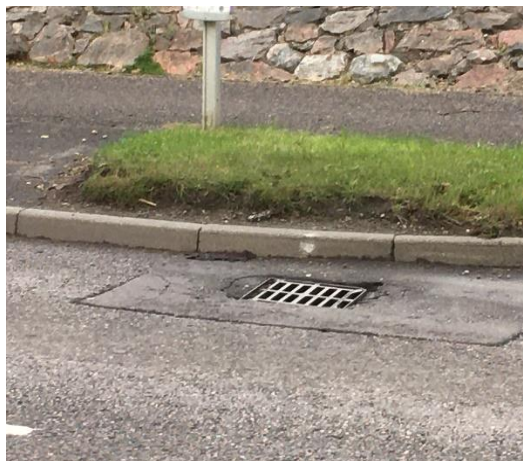
Sunken drain cover at Kilmallie Gardens bus stop.
