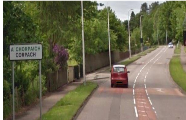
Corpach signage travelling West. No indication that Corpach is a residential area. Poor faded road markings.
