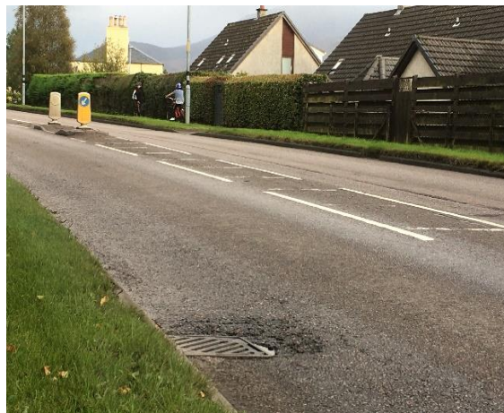
Sunken drain cover close to Hillview Drive.
