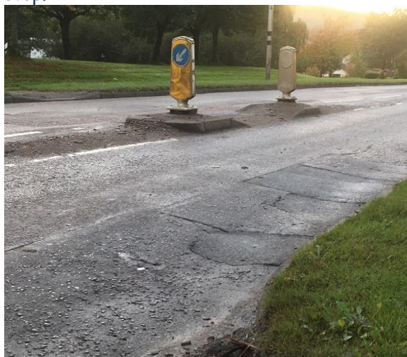
Traffic island by Kilmallie Gardens. Poor and sinking road surface.
